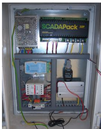
Figure 5. RTU SCADA board
